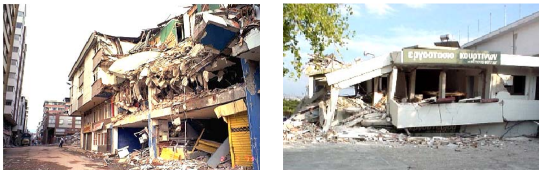
Figure 4s. These RC structures did not withstand earthquake forces during the January 1999 Armenia, Colombia and August 1999 Athens, Greece tremblors. (Source: Scawthorn, 2000.)
